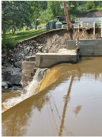
Damage to Right Abutment Contact
