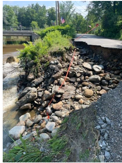
Damage to Left Abutment Contact
